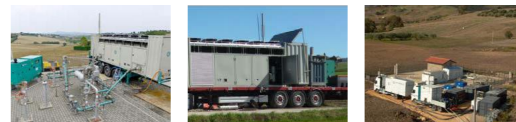
Mobile compressor - Snam gas facilities
