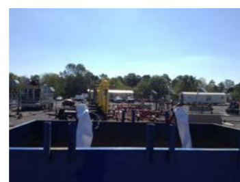
Flow lines move gas to separator which removes free water from natural gas and delivers the natural gas into the meter and pipeline.
