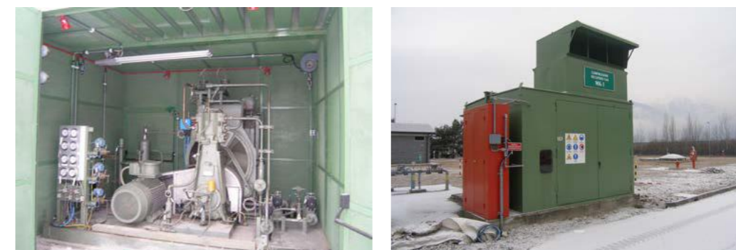
Gas recovery system installed in Snam compressor stations
