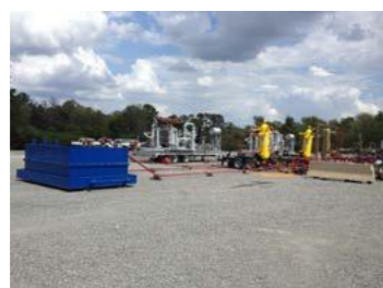
Temporary Equipment Associated with Gas Capture or Green Completion methodology. Gas compressor located on portable trailer (center of photo) and may be used for initial gas lift. Choke manifold is "red piping and valves" used to control flow from the well. Vertical sand separators (yellow) – separates sand from water and gas. Sand is directed to the blue storage container. Gas and water are routed to separator with gas going to pipeline and water going to storage.
